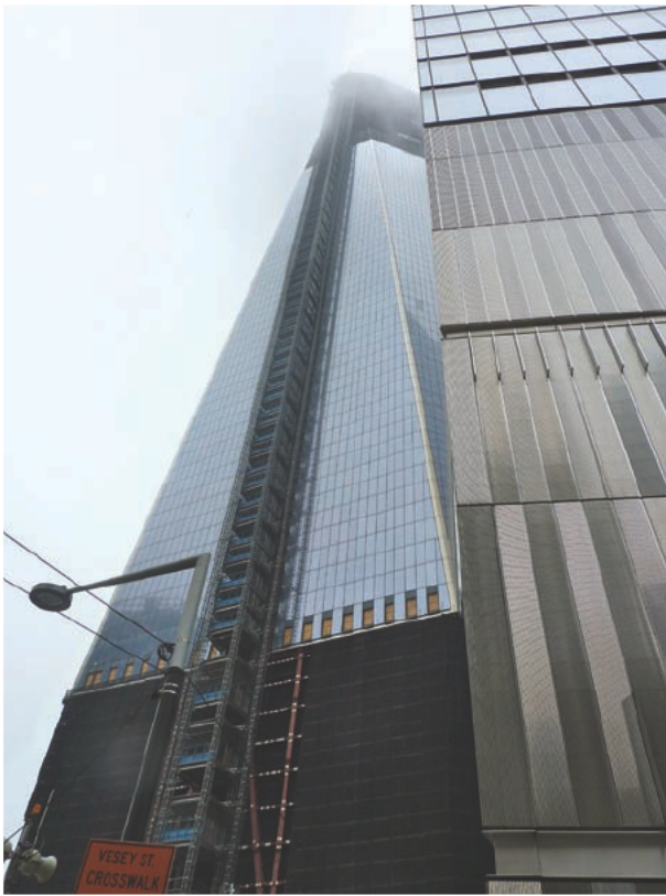
◀ Freedom Tower under construction at the World Trade Center site in New York City. When completed, the tower will stand 1,776 feet tall and be surrounded by several other buildings, and a memorial to the nearly 3,000 people who were killed in the terrorist attacks that demolished the Twin Towers in 2001. How did those attacks change the American justice system? Courtesy of The Justice Research Association
